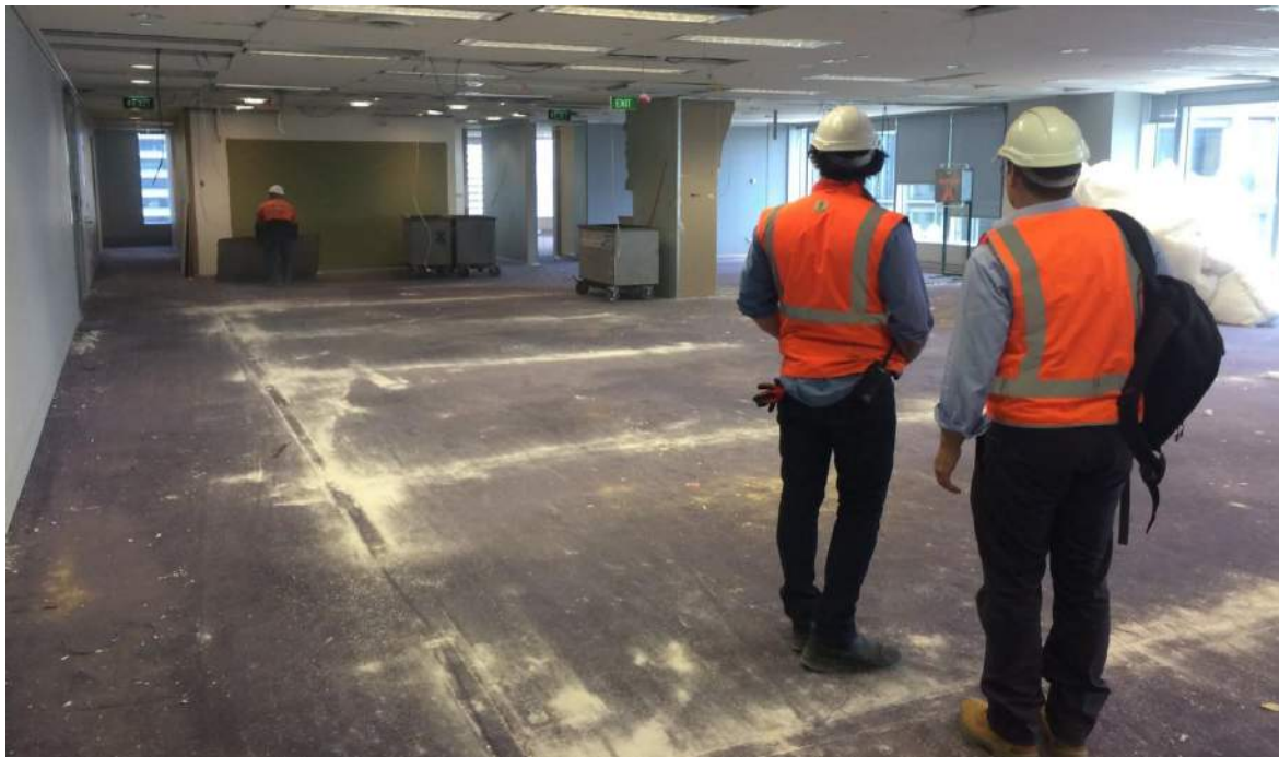
Structured demolition of Levels 34--41 underway – furniture, gypsum board and stud walls, glass and cabinetry removed. Broadloom carpet and ceiling tiles still remain.
